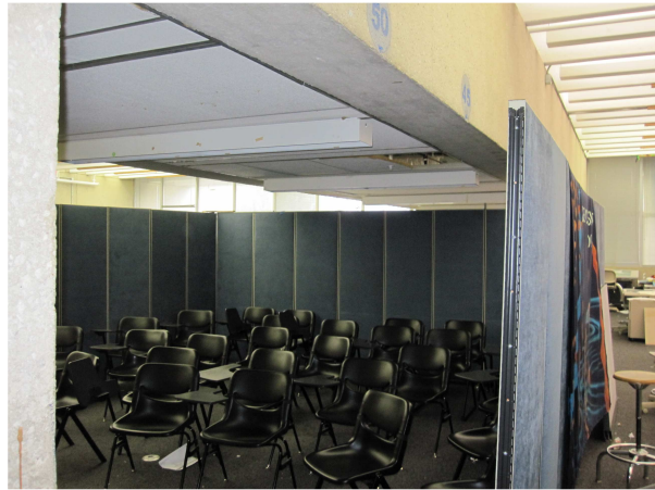
Partition walls of the west side of the review space. Note the ceiling/lighting is in poor conditions. The wall is also tilting.
